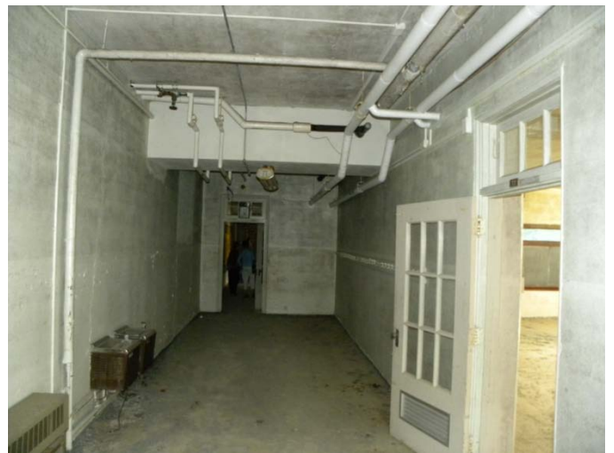
I wonder how much asbestos and lead based paint is in the building?
