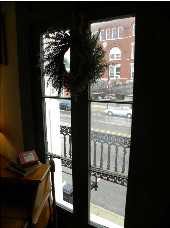
The floors to the balconies are missing
